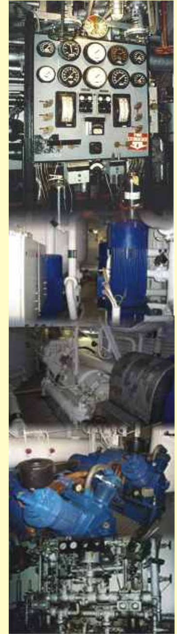
Control room Cooling water system Feed water system Turbo charge Engine room
